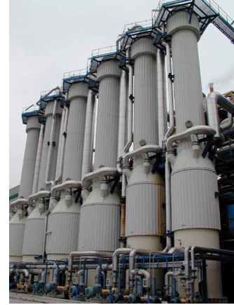
Figure 1. Five evaporation units for the evaporation section in a beet sugar factory in Spain.
